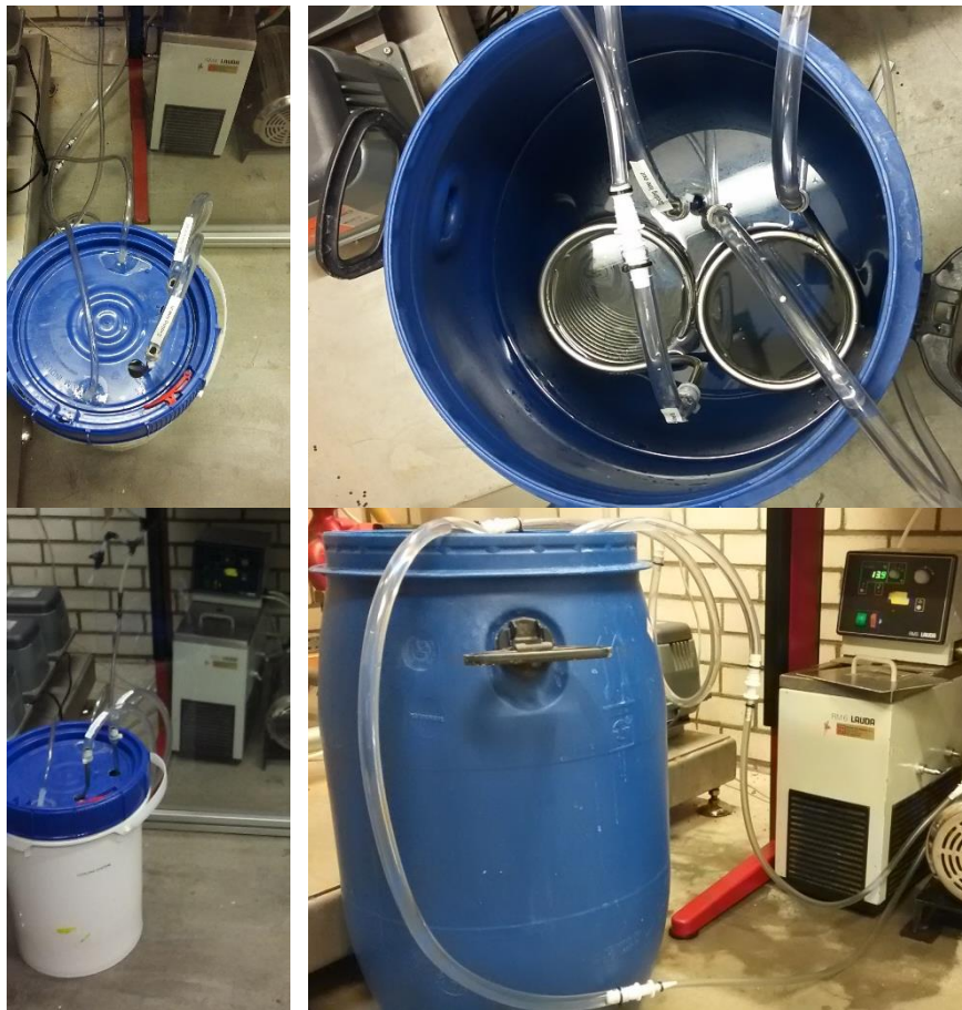
Figure 5-18: On the left, the cooling system; on the right, the installed one.
