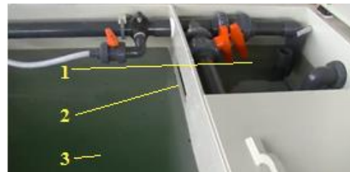
Figure 13: Anoxic tank (1). After this compartment, the effluent reaches the aerobic zone (3) by an overflow (2)
