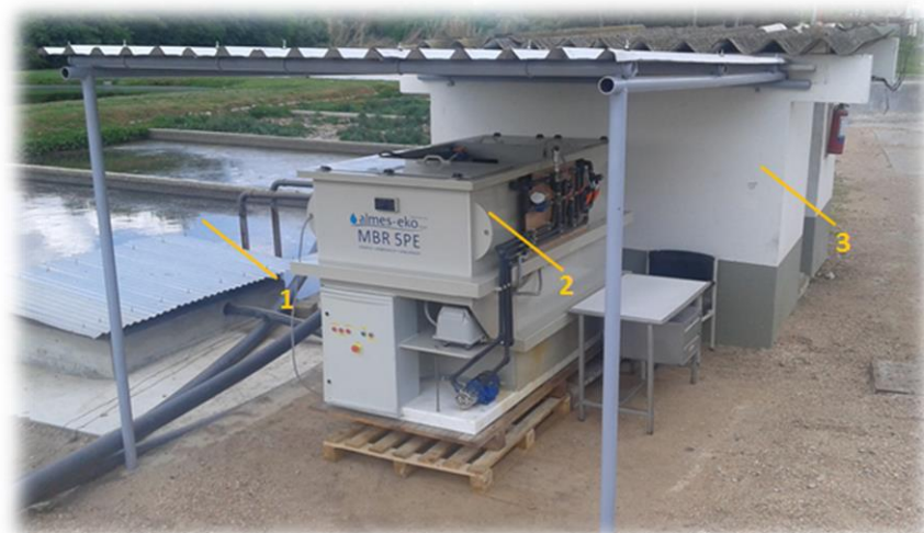
Figure 19: Inlet from homogenization basin (1); MBR (2); Room for electric panel (3)
