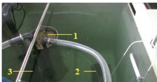
Figure 14: Aerobic tank, with immersed membranes (1), a diffuser for providing air (2) and a recirculation pump (3)
