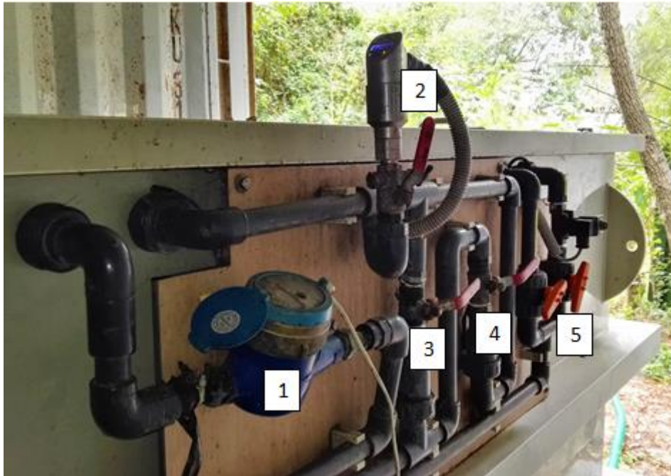
Figure 5 Pilot scale MBR valves system and control elements.1-Flow meter; 2-Pressure sensor; 3-Backwash valve; 4-Permeate valve and 5- Air valves.
