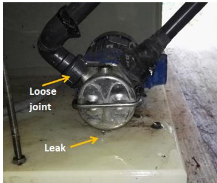
Figure 26 Leaking reversible pump
