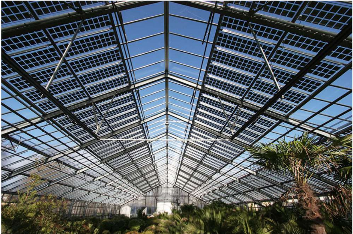
Figure 3.23 Building Integrated Photovoltaics (BIPV)
