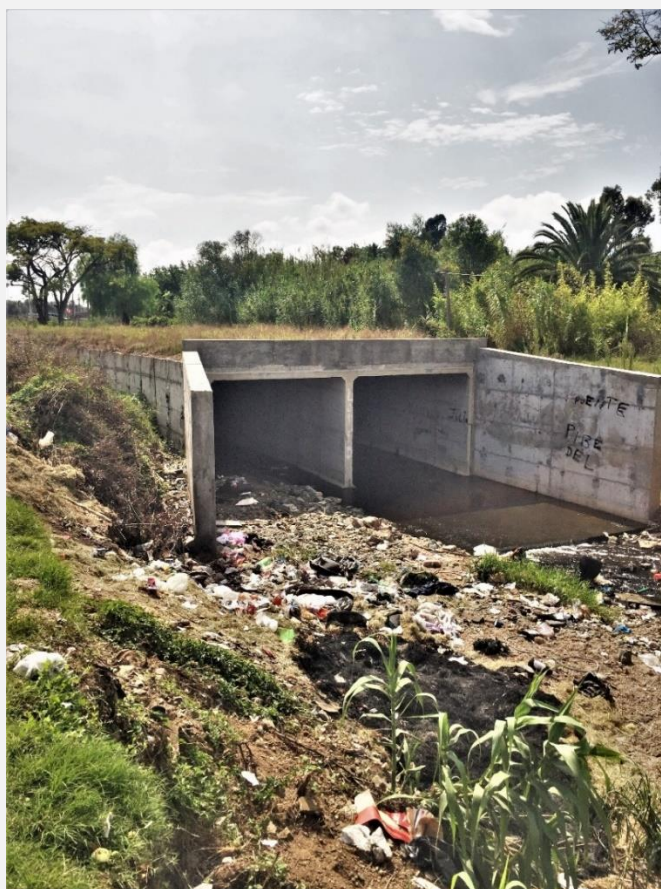
Figure 2.14: Road and sanitation work at Iyú Stream and San Martín Avenue intersection. Date: February 2022
