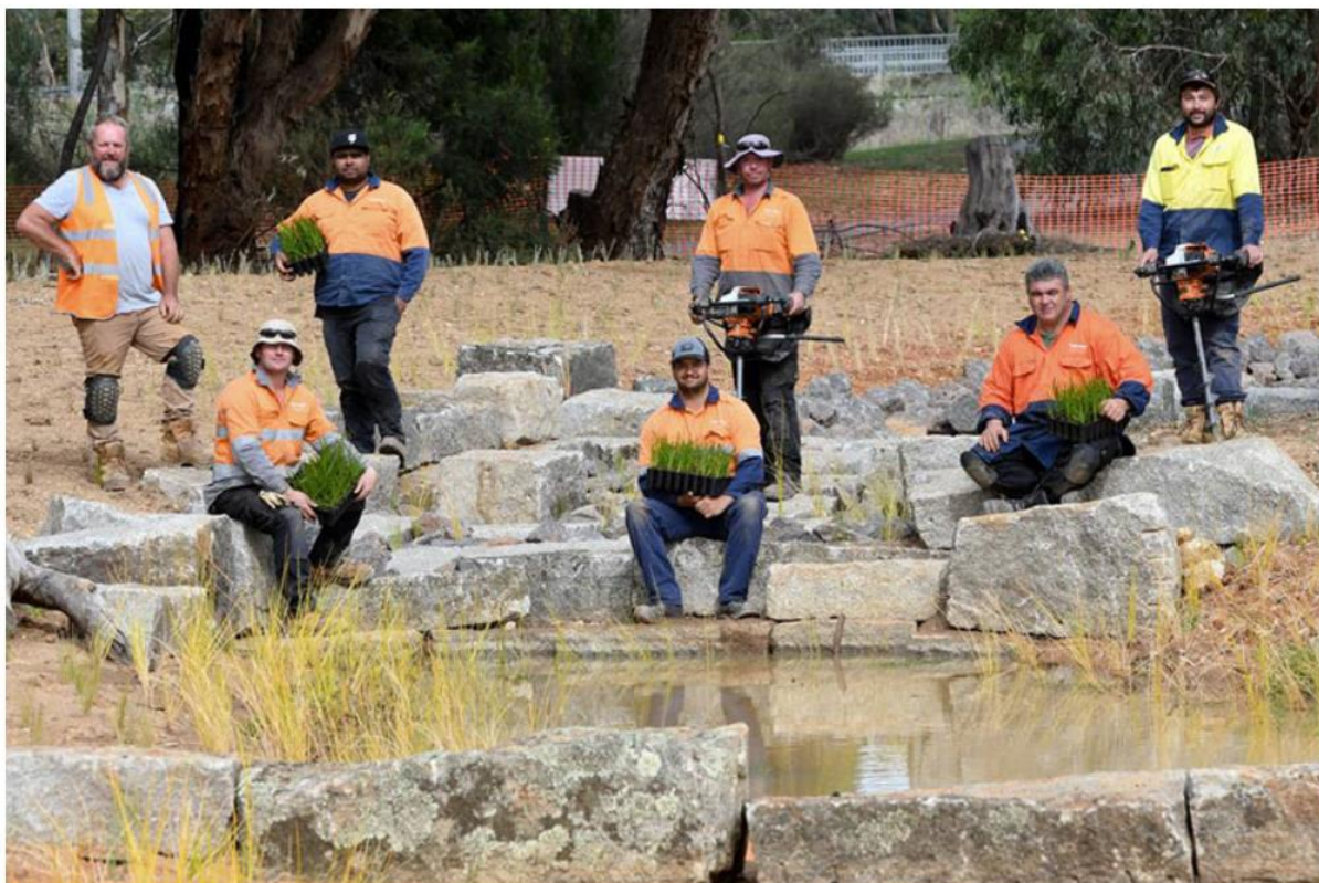
Figure 0.4.14: Djandak team members at Koomba Street's new project healing storm water before it flows into the Bendigo Creek.
